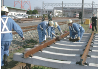
Training for track damaged
