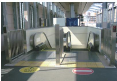
Escalator at Kashii-Miyamae Station
